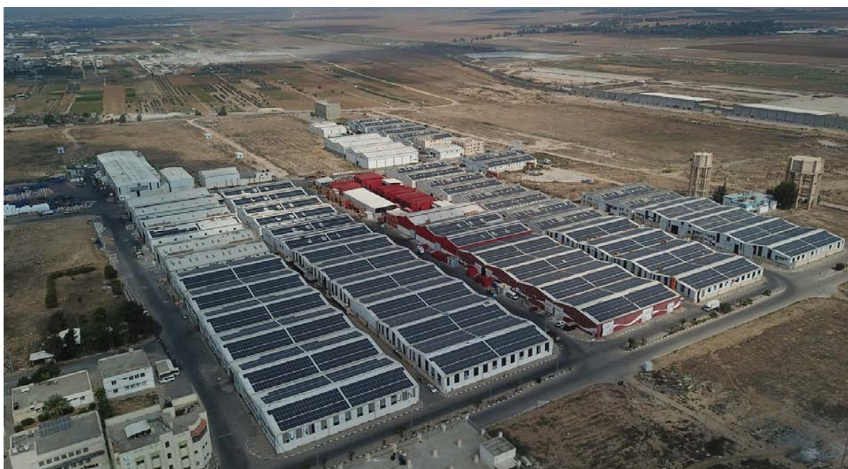
Figure 4: Solar photovoltaic panels installed at the Gaza Industrial Estate, part of an IFC-funded project on renewable energy in Gaza, which was recognized as an important example of “Financing for climate friendly investment” (Source: World Bank Group)
